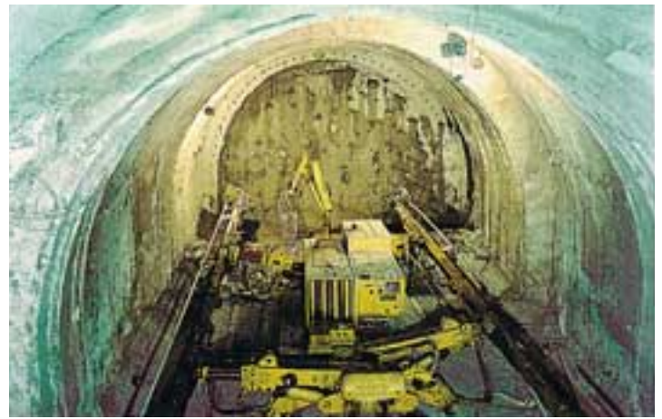
Photo 3: Vasto Tunnel: reinforcing of the advance core with fibre-glass tubes during full face excavation (according to A.DE.CO.-RS principles).
