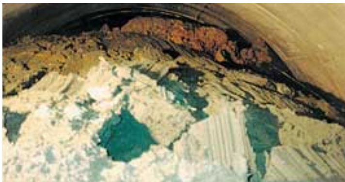
Photo 2: Vasto Tunnel (Italy, Ancona to Bari Rail Line, ground: silty clay, overburden: 135 m, tunnel diameter: 12.20 m.). The extrusion of the ground through the face during heading and bench excavation (according to NATM principles).
