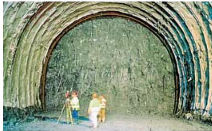
Photo 5: Pianoro Tunnel (Italy, Bologna to Florence High Speed Rail Line, ground: cemented silty sand, overburden: 150 m, tunnel diameter: 13.30 m.). View of the face reinforced with fibre-glass structural elements.
