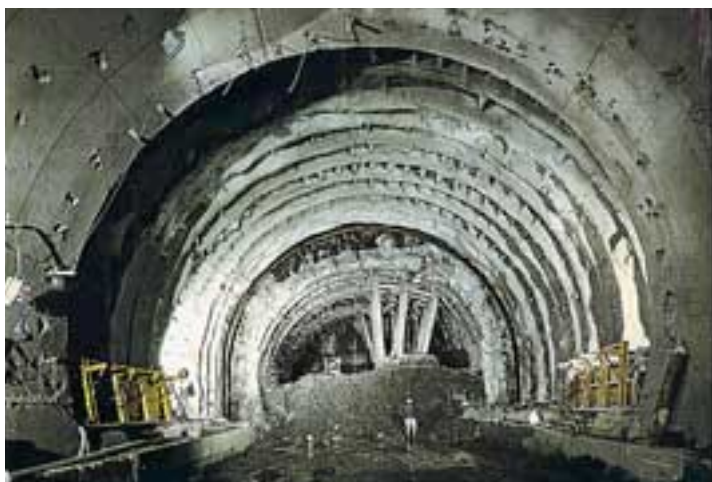
Photo 1: S. Stefano Tunnel (Italy, Genoa To Ventimiglia Rail Line, ground: tectonised and laminated marly-limestone flysch, overburden: 150 m, tunnel diameter: 12 m.). Collapse of the cavity.
