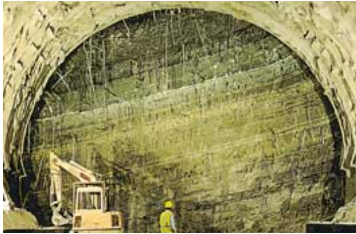
Photo 4: Tartaignulle Tunnel (France, Marseille to Lyon TGV Méditerranée, ground: swelling clay (75% montmorillonite), overburden: 100 m, tunnel diameter: 15 m.). View of the face (180 m²) reinforced with fibre-glass structural elements.
