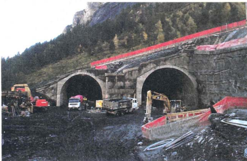
Northern portals of the twin-tube Dolonne tunnel on the Aosta-Mont Blanc motorway.
