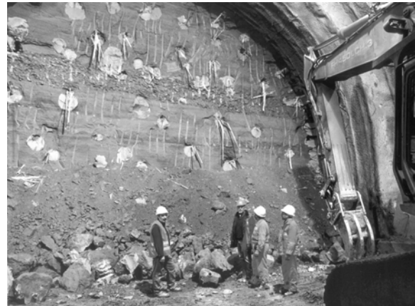
Figure 6. Firenzuola tunnel: the face reinforced with fibre glass structural elements inserted into micro jet-grouted columns
