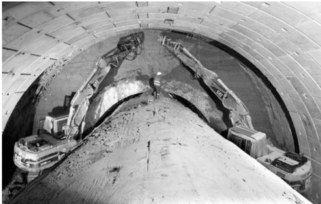
Figure 8. The demolition of the widening face performed using two road header excavators.
