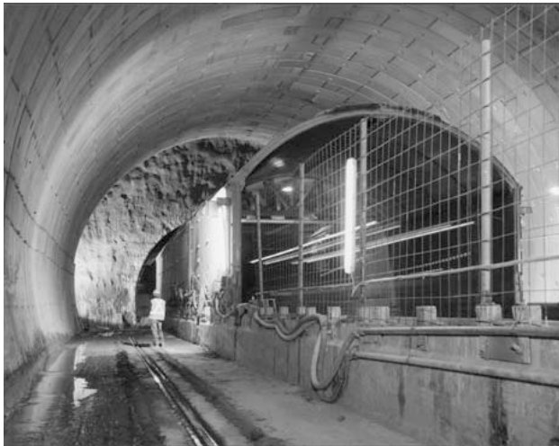
Figure 7. The steel shield to protect traffic.
