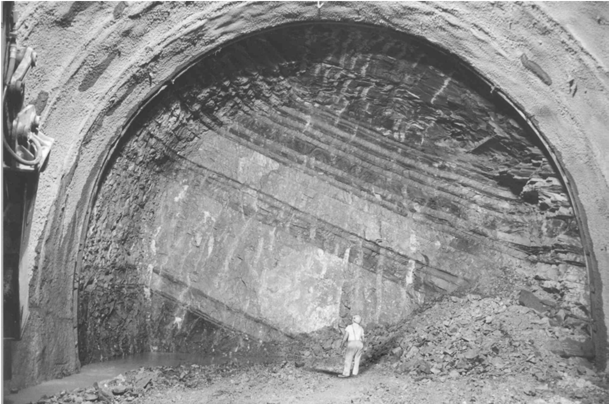
Figure 7. The face of the Vaglia tunnel in the Monte Morello Formation (limestones, marls and sandstones )
