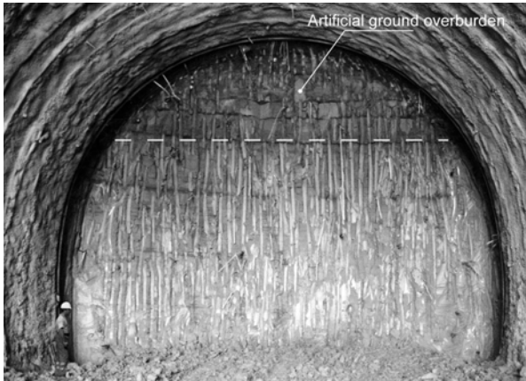
Figure 6. Borgo Rinzelli tunnel: the face during the advance under artificial ground overburden
