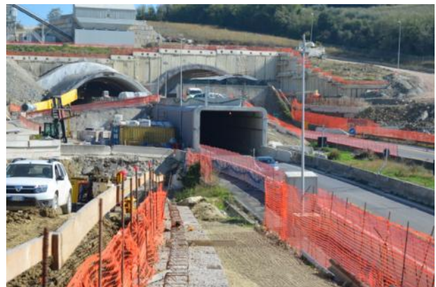
Figure 8. Montedomini tunnel: traffic protection shield
