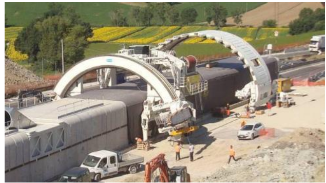
Figure10. Montedomini Tunnel: the two machines used to widen the tunnel in the presence of traffic
