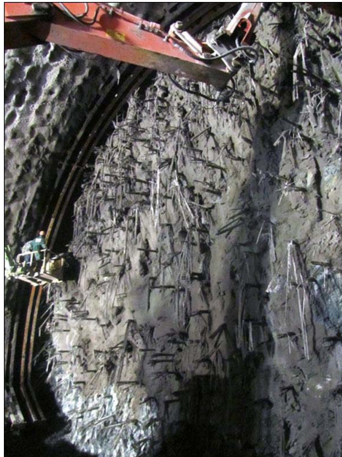
Figure 8. Face of the T8A tunnel – North portal in the landslide area – slope deposits
