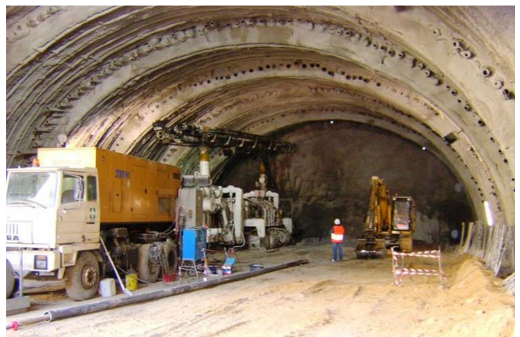
Figure 23: Enacting reinforcement of the core-face for the C1 section type, it is also visible the crown treatment with compenetrated jet-grouting columns reinforced with steel tubes
