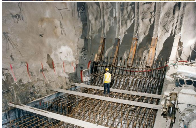
Figure 14. Invert cast at the excavation face – Raticosa Tunnel ( \varnothing = 13.90 \text{ m} , Ground: scaly clays, Coverage: 500 m) and Tartaguille Tunnel ( \varnothing = 15.30 \text{ m} , Ground: expanding clays, max Coverage: 150 m).
