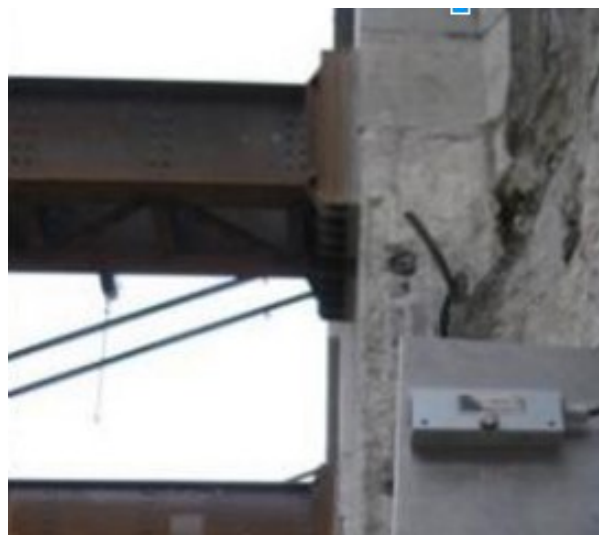
Figure 10 Surface electro-levels monitoring
