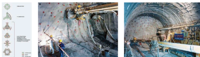
Figure 3. Fiber glass element profile Core face reinforcement execution insertion and execution drilling of the fiber glass element.
