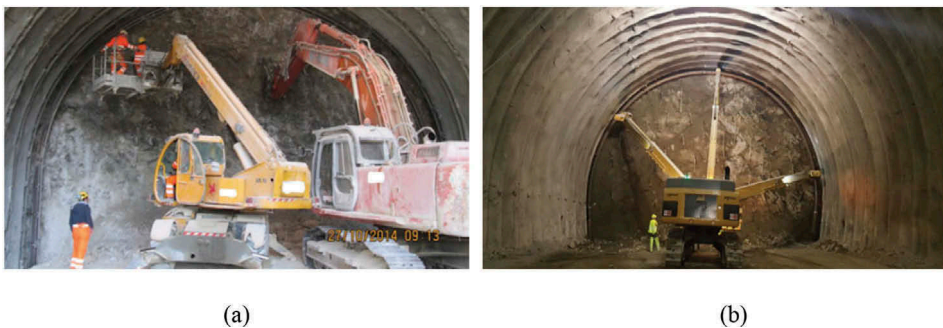
Figure 7. (a) Traditional steel rib installation method. (b) Semi-automated steel rib installation method.
