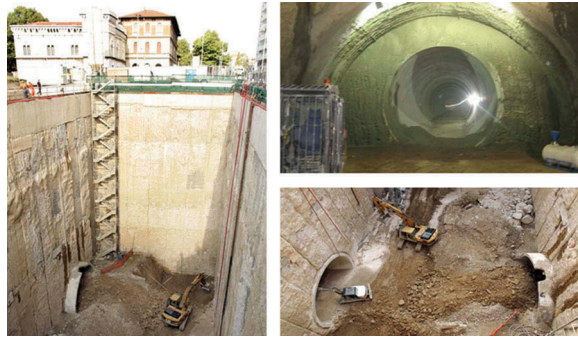
Figure 10. Work Phases: the excavation of the station shaft and of the tunnel station.
