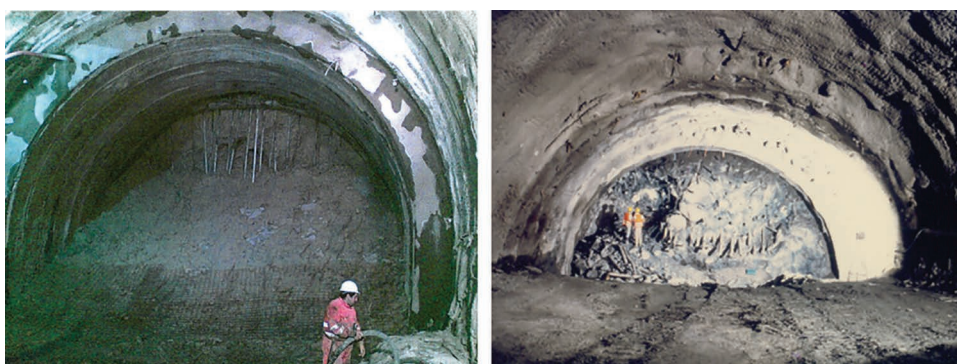
Figure 4.8 Examples of the failure of the umbrella arch due to the absence of the first rib. This mistake contrary to the design requirements resulting in bending the steel pipes and tunnel collapse.
