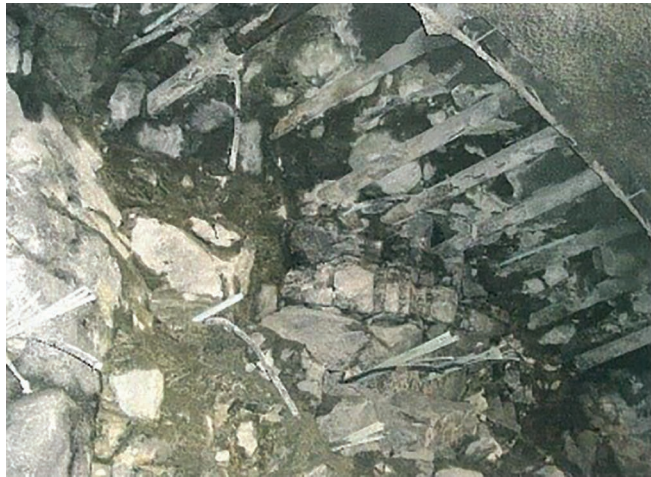
Figure 4.10 Example of a too long excavation. The excessive length of excavation can determine an excessive load on the end of the excavated span and it has caused the collapse of the face, followed by the collapse of the pipes.
